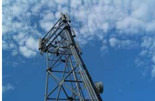
Typical Greenfield - Tower
