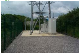
Typical Greenfield - Cabs
